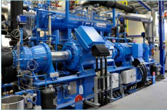
figure 11: One of the heat pumps at the steel and rolling mill Marienhütte (Energy Graz)
