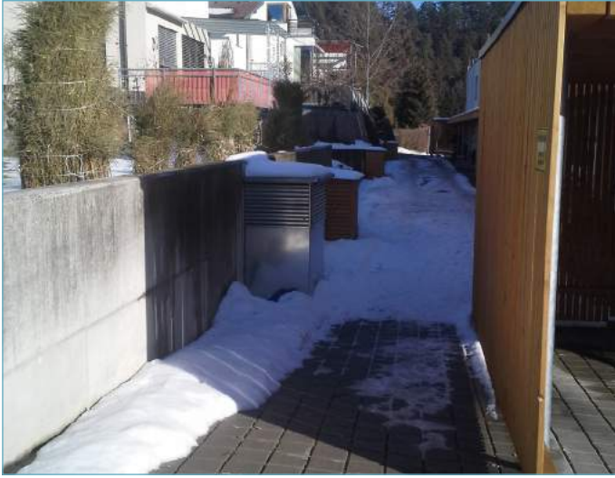
figure 14: an installed heat pump at one of the houses (Kleboth & Dollnig)
